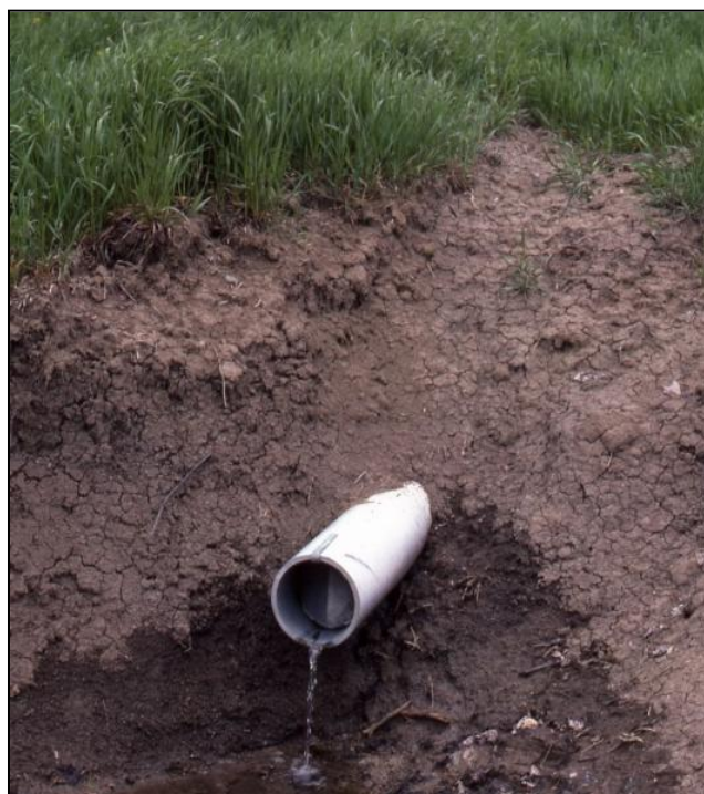
Figure 1: Clean water exiting a modern tile drain.
